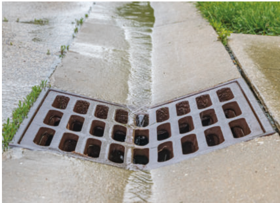
Rain runoff on the roadside (Source: JJ Gouin|stock.adobe.com)
