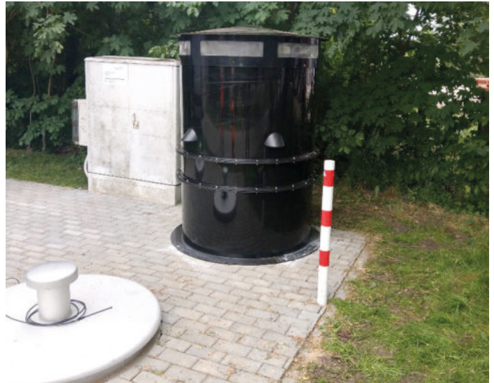
Filter for removing odour from exhaust gas in a sewage tunnel (Source: HeGo Biotec GmbH)
