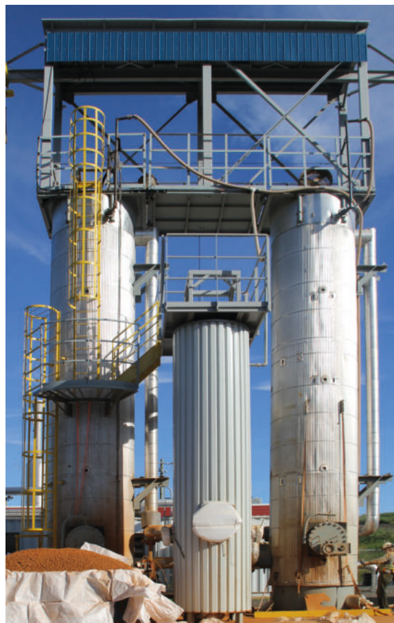
Landfill gas application, Quebec, Canada (Source: HeGo Biotec GmbH)
